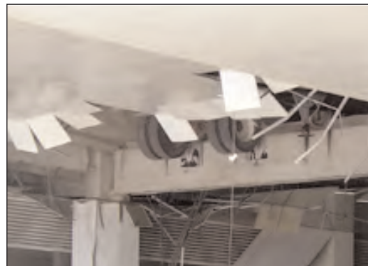
On the first day of the conference, a section of the concrete floor in the loading dock at the David L. Lawrence Convention Center gave way under the weight of a tractor-trailer resulting in the evacuation of the center...
